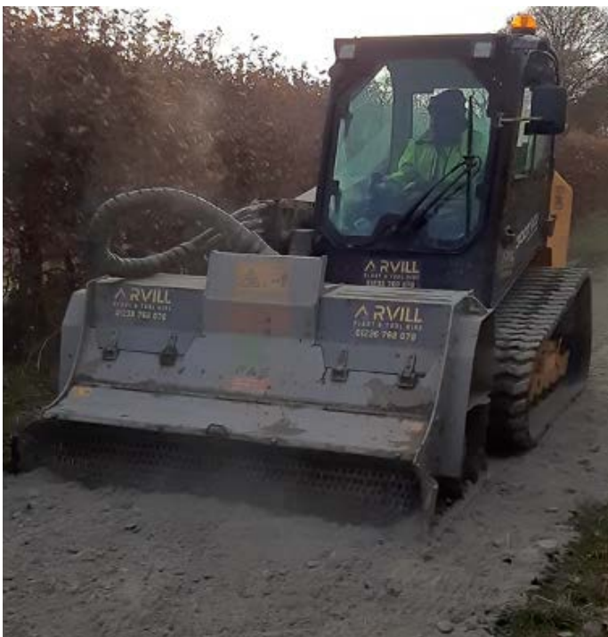
Figure 3 – Smart Surface powder being mixed into the soil using Skidsteer Mounted Crusher
